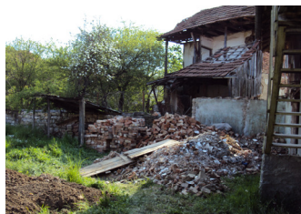
Heaps of bricks and old building materials. We kept the usable stuff. The rest is gone now.
